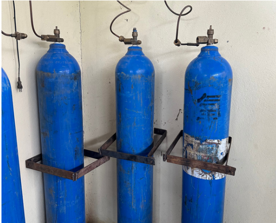
Brackets keeping oxygen cylinders in place
